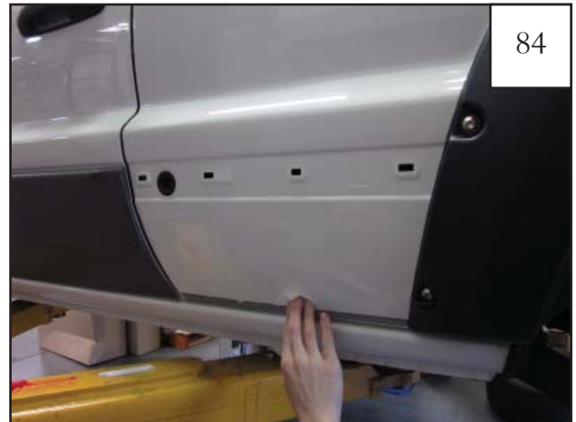
Prior to re-installation of the cladding, use a supplied alcohol prep pad to clean the sheet metal and any factory tape residue.
